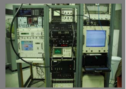
Control Room at 21 M
