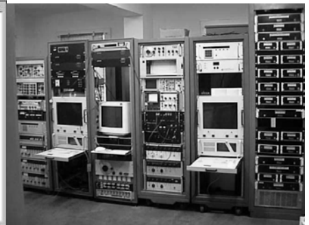
Control Center at SSC
